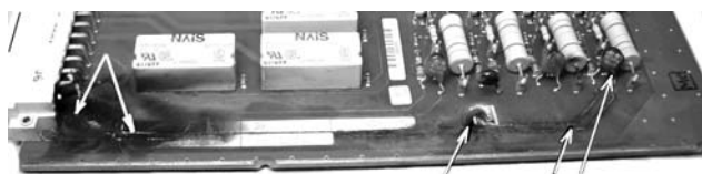
Fig. 6. Fragment of I/O module with numerous damages elements and breakdown tracks on printed circuits.
