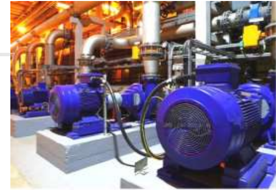
Induction motors - the driving force of the pump stations
